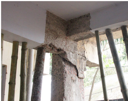
Fig. 1. Severely damaged column in ground floor. One column in the ground floor damaged severely. Big shear cracks and concrete spalling were found at the top of the column.
