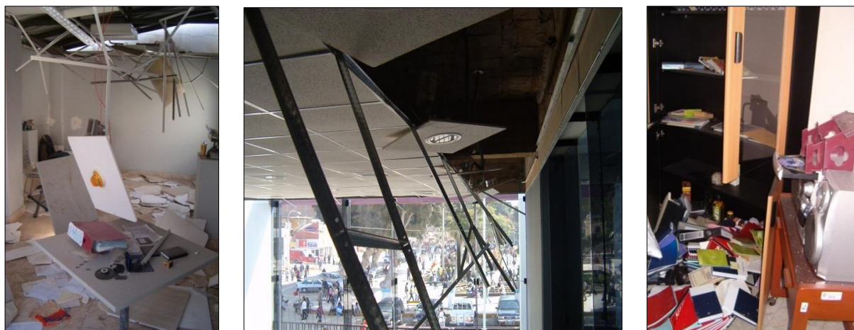
Fig. 15. Three story R.C. Custom building in Pisco with non-structural damage and in its content. Photos kindly provided to the author by the administrator of Pisco Custom Office.
