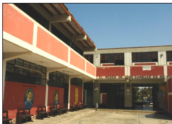
Fig. 13. Left block designed with Peru Seismic Code of 1977 and right building with the 1997 version. Photo taken by the author in Ica. September 2007.
