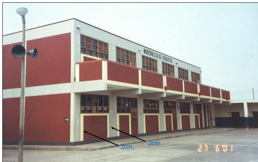
Fig. 14. Safe Peruvian school building in the Arequipa Region, Peru. Photo taken by the author, June 2001.
